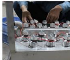
5 Sky men Transducer Wiring
